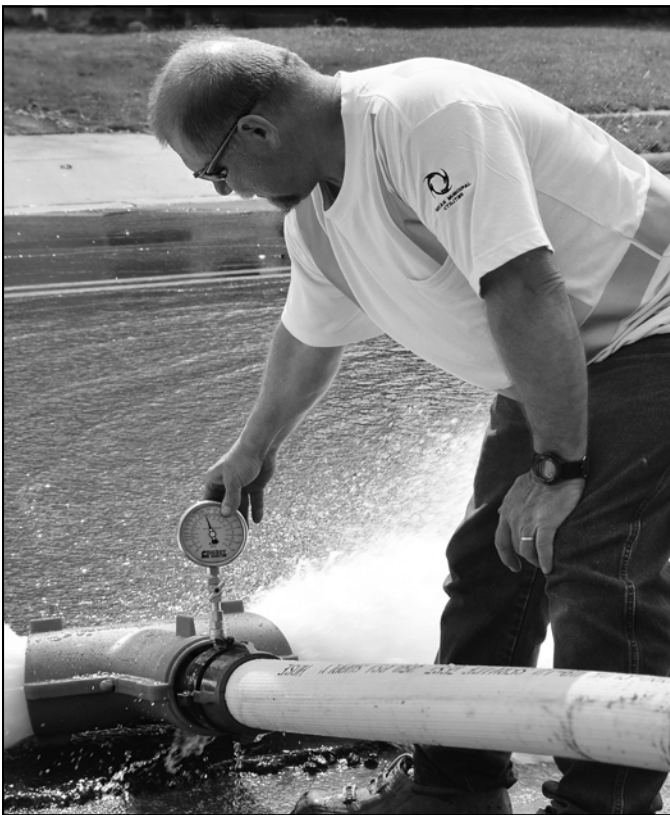
Water Operator Eugene Wilson checks flows and pressures as part of our annual system flushing and hydrant inspection.
