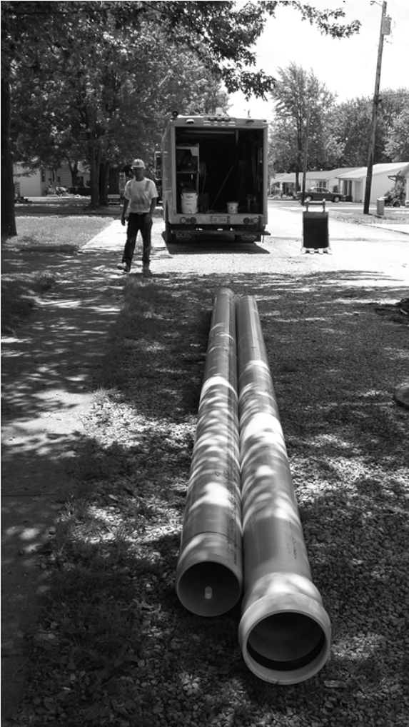
Water department workers prepare to install new eight-inch water main on South Myers Street.
