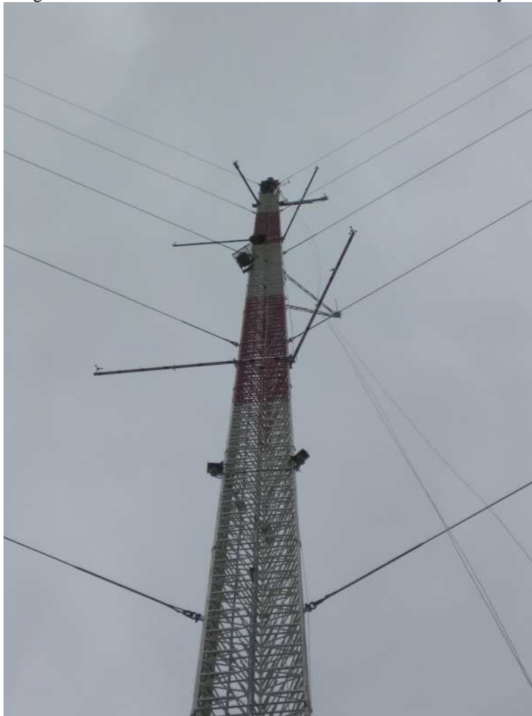
Figure 2: Instrumented Booms on Communications Tower at Bryan
