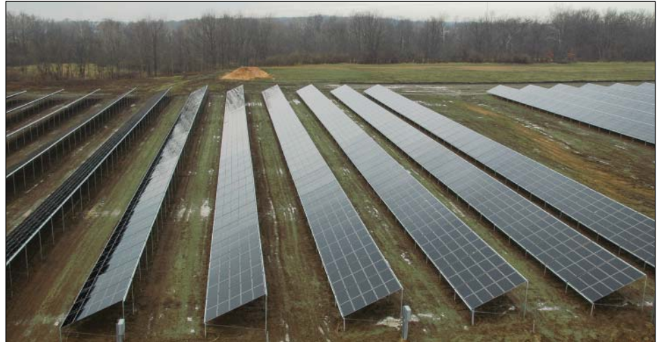
Bryan's new solar array, located just west of Bryan on State Route 34, supplies power directly to the city's electrical grid.
