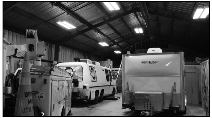
New energy efficient T-8 lamps in the communications warehouse.
