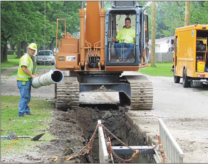
Water Supervisor Nate Gardner guides a piece of water pipe into the trench as operator Jeff Grant assists with the excavator.
