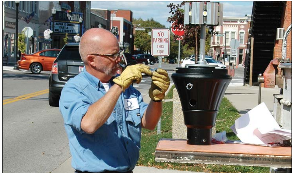
Lineworker Kyle Robinett prepares one of Bryan's new energy-efficient LED historical lights for installation. Energy savings on the new lights is about 50 percent.
