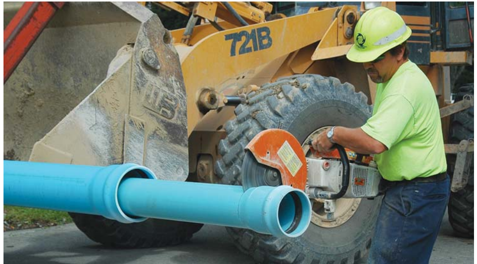
Water Operator Gus Hulbert cuts a piece of waterline to length for Clover Road.
